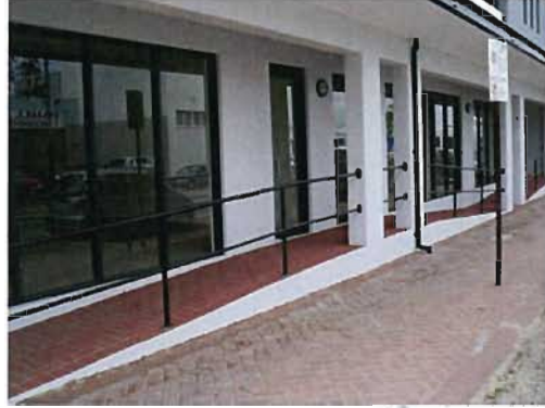
A difference in levels between the public footpath and the front door of this building has led to this unnecessary and clumsy design result.
