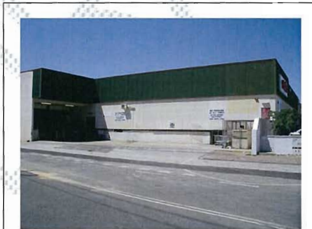
This service loading dock is located on a street front. The facility is visually unattractive, noisy and creates a very poor environment for passing pedestrians. It also includes a 20m-wide crossover used by reversing trucks which is potentially dangerous for pedestrians. A facility designed in this manner will not be permitted.
