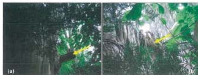
Figure 2. (a) A branch stub resulting from previous indiscriminate lopping (see arrow) was visible at 1.5m on the south side of the tree; (b) A mud gallery encasing probable active termite infestation was evident (see arrow) on the tensile side of the attachment of the first order structural branch at the crown break approximately 2m above ground level; looking towards the north-east.
