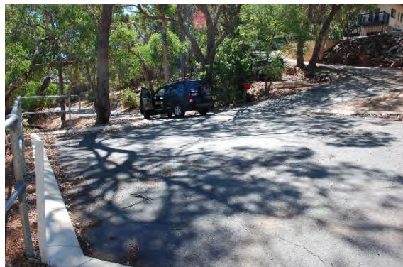
Small turnaround area does not comply with current standards.
