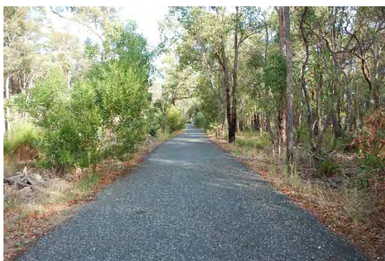
Narrow road – does not comply with current standards
