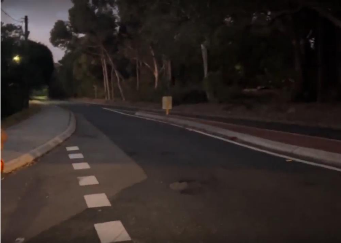
Photo 13: Poor lighting on the north leg of Elizabeth St/Railway Rd intersection
